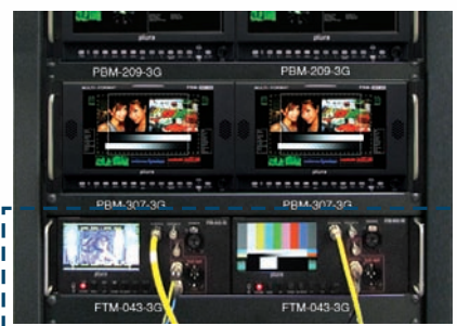
(2) FTM-043-3G units in Rack Mount - 2RU
